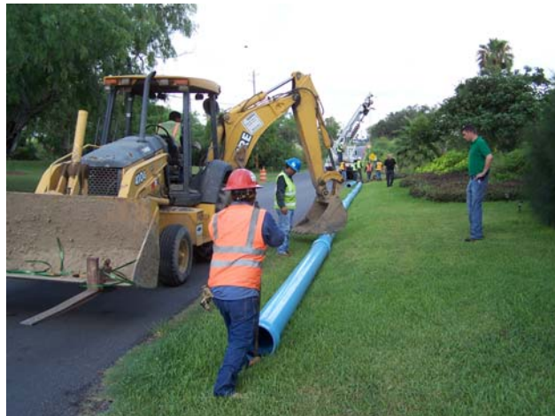
The backhoe's bucket center loads the previously installed length of pipe to keep it from moving while the new joint is being assembled.
