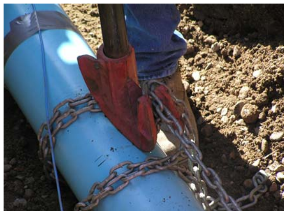
This assembly tool uses a chain wrapped around the bell and a lever bar to make the joint.
